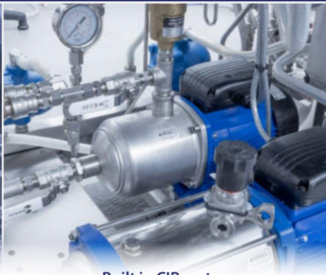
Built in CIP system
